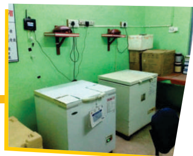
Deep Freezer running through solar power
